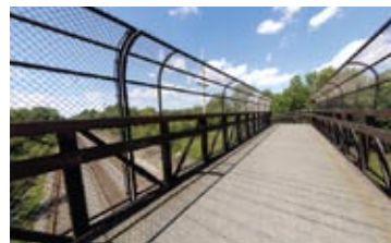
A grant from The Burton D. Morgan Foundation provided this elevated footbridge that crosses the railroad tracks near South Hayden Parkway.
